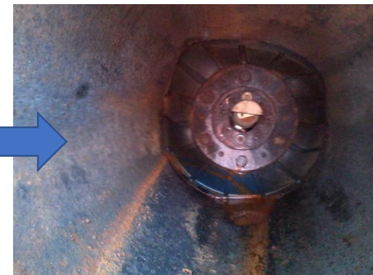
Damaged Section Cut Out
