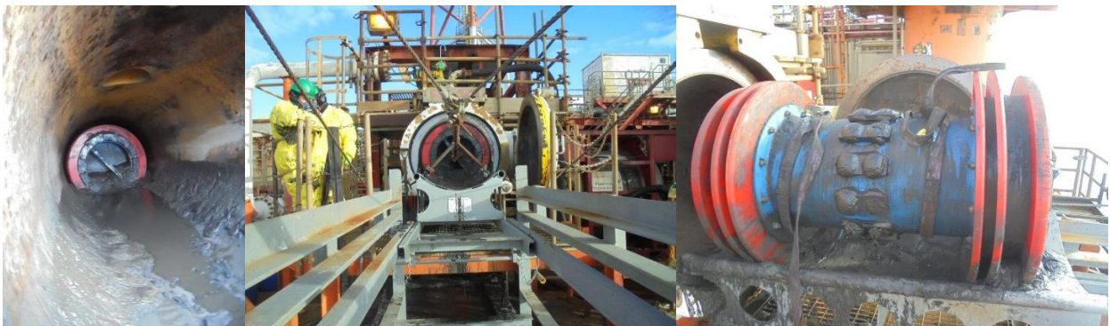
Figure 7: 36-in., 118.7-km Gas export pipeline offshore pig receipt
