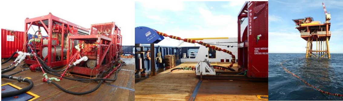
Figure 5: Supply vessel-based flushing spread complete with flushing 2-in. high-pressure (HP) hose deployed to satellite platform
