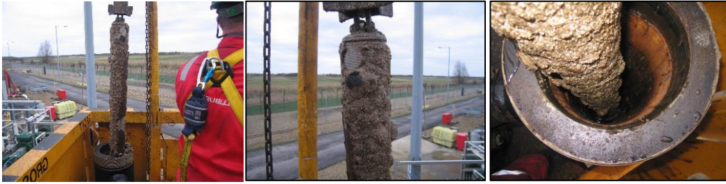
Figure 4: Debris removed from 4-in., 118.7-km methanol pipeline
