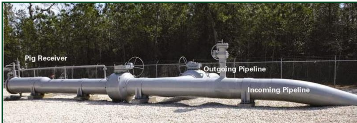
Typical Onshore Pig Receiver
