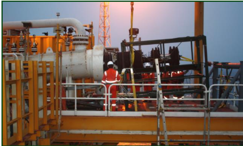
PLR Operations – Pig Loading
