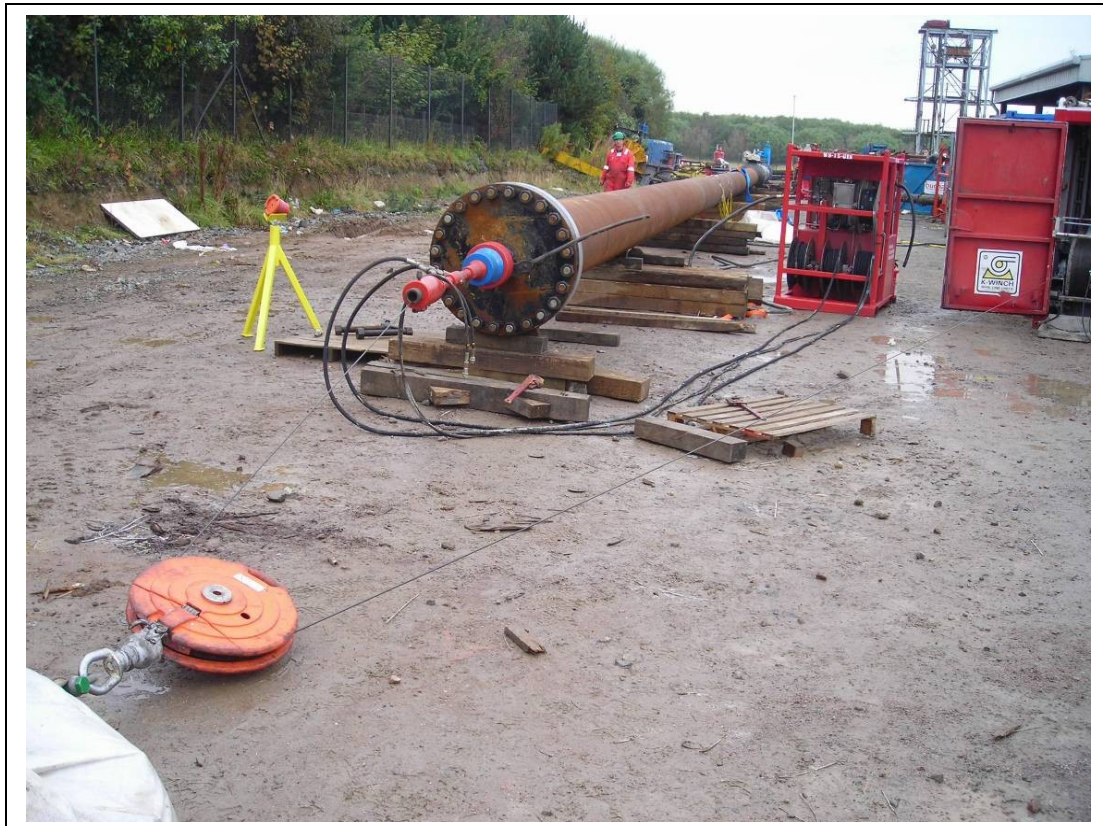
Figure 8 - Hoop Stress Testing
